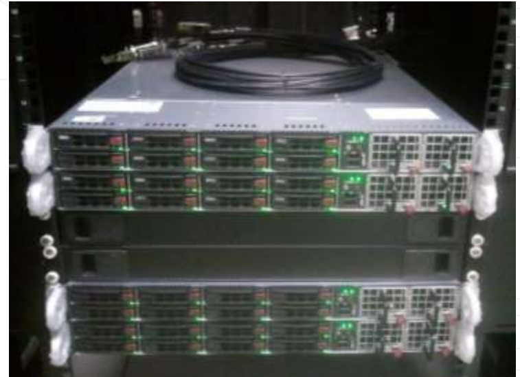
Kaminario 6TB all flash array
