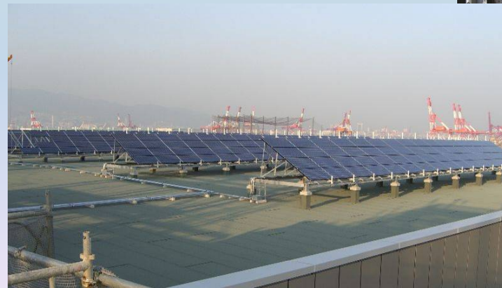
Solar panels on the top
