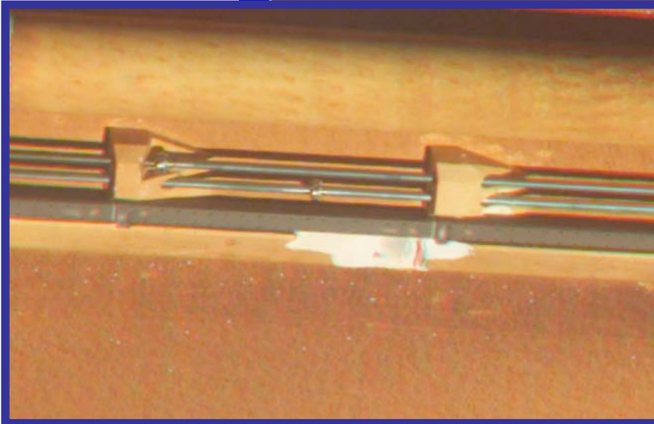
Area of LH2 PAL ramp missing foam
